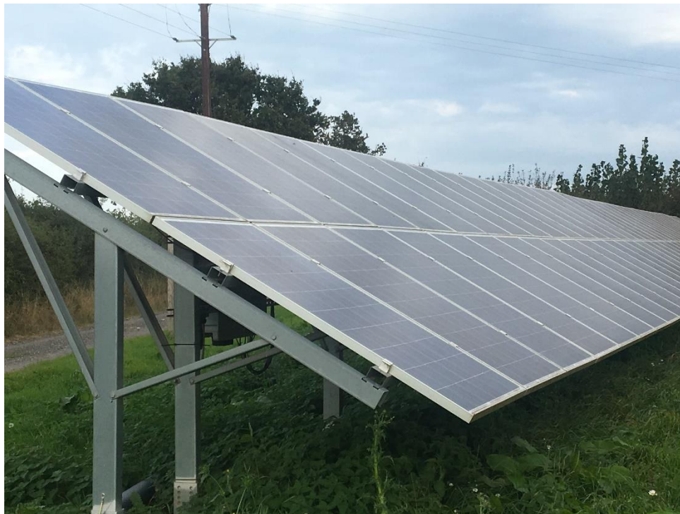
Plate 2-3 Solar panels with south facing configuration
